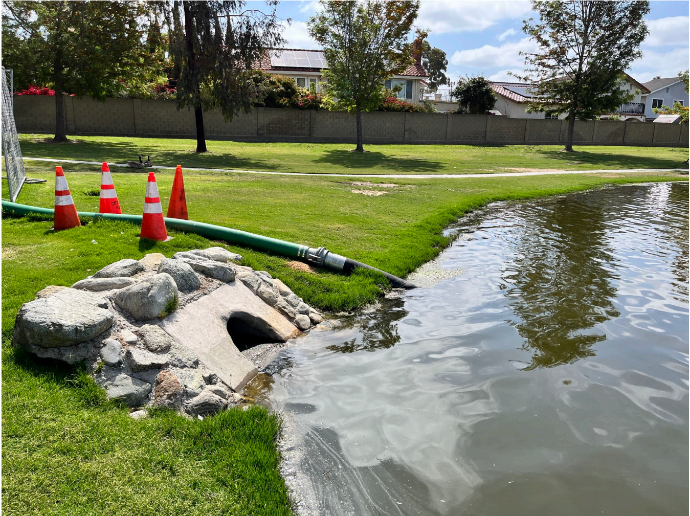
Figure 1-8. Lake outlet structure and emergency evacuation pump line at Greer Park South.
