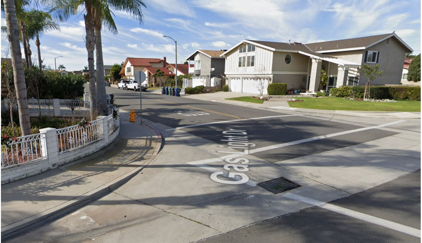
Figure 1-5. Water marks past the curb due to inadequate drainage near the intersection of Dawson Ln and Gas Light Dr.
