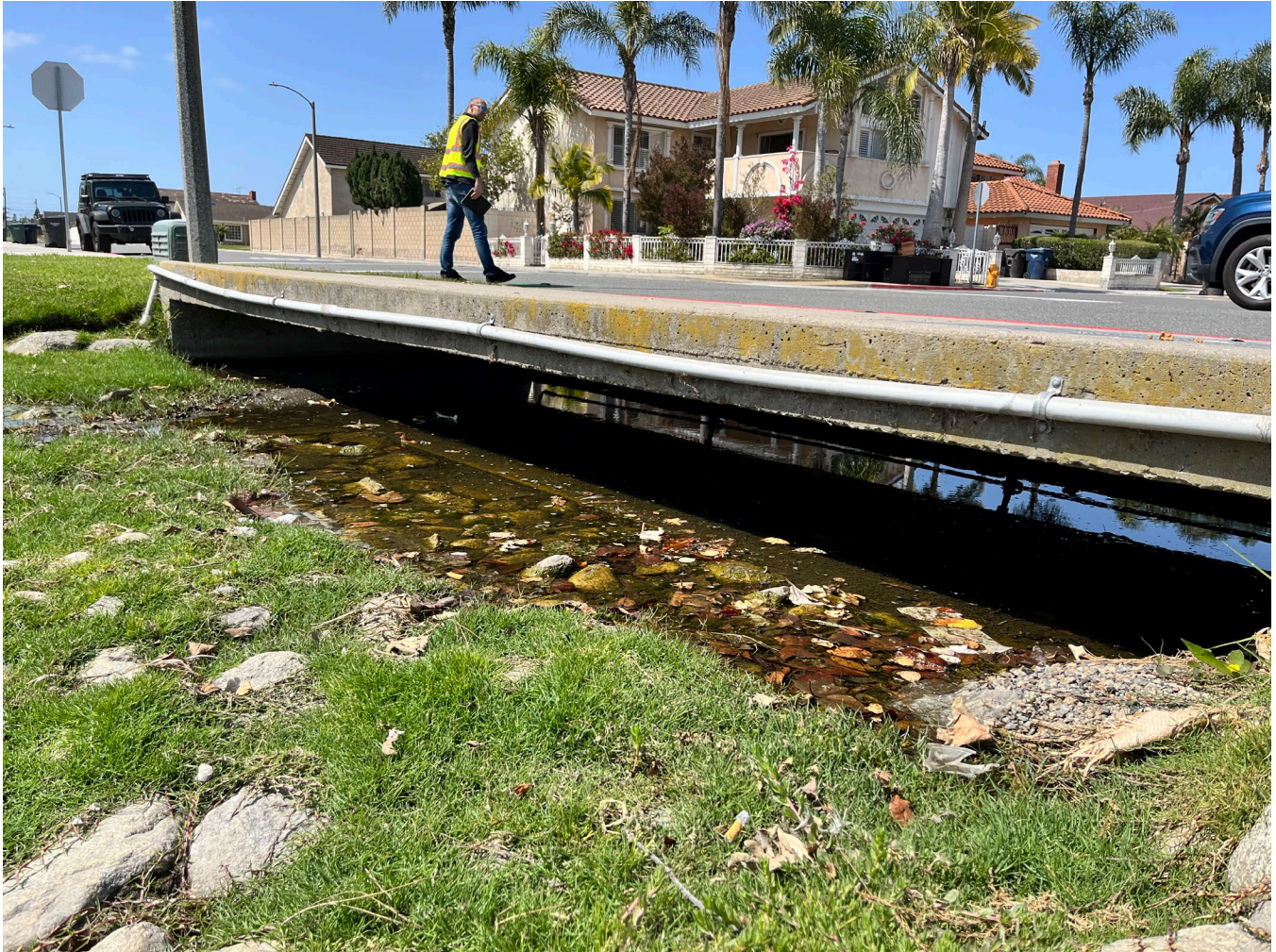
Figure 1-4. 16' curb inlet at eastern side of intersection of Dawson Ln and Gas Light Dr.
